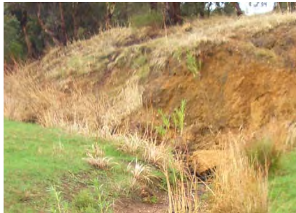
Plate 1: Heavily eroded bank on northern side of Beenyup Brook
