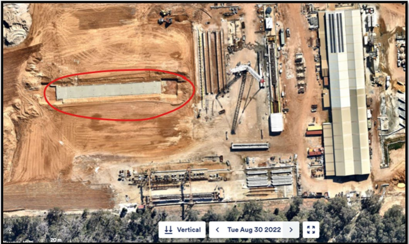
Image 2: 30 August 2022. Note new stressing bed being built with no Shire or DWER approval. Located close to the western boundary, and orientated in such a way that noise is directed on an east west direction
