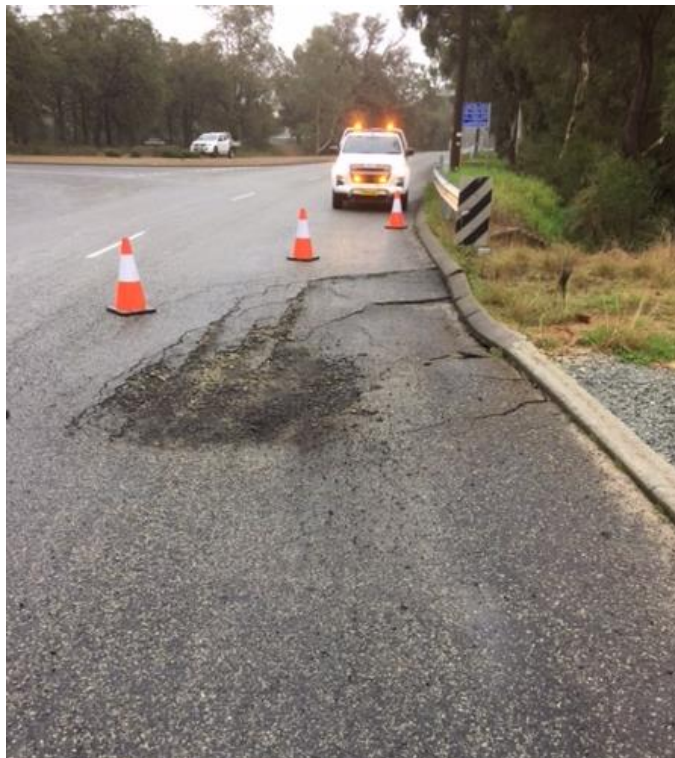
Photograph 6: Historical photo (provided by the Shire) showing subsidence of the northern end road surface
