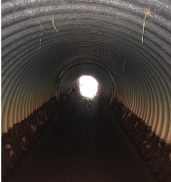
Photograph 5: Separation and failure of the joint from the southern end
