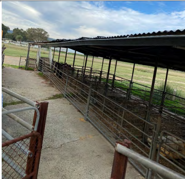
Parts of the roof buckled
