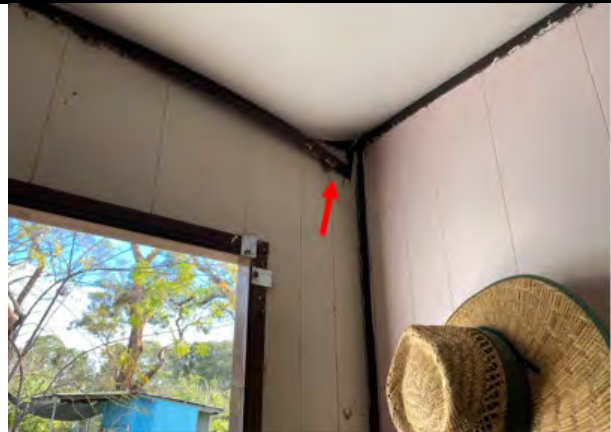
Ceiling sagging and damage
