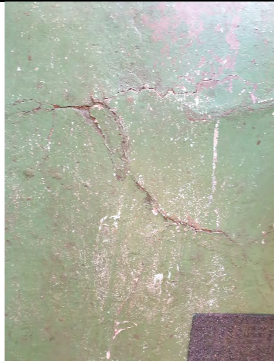
Crack in concrete slab
