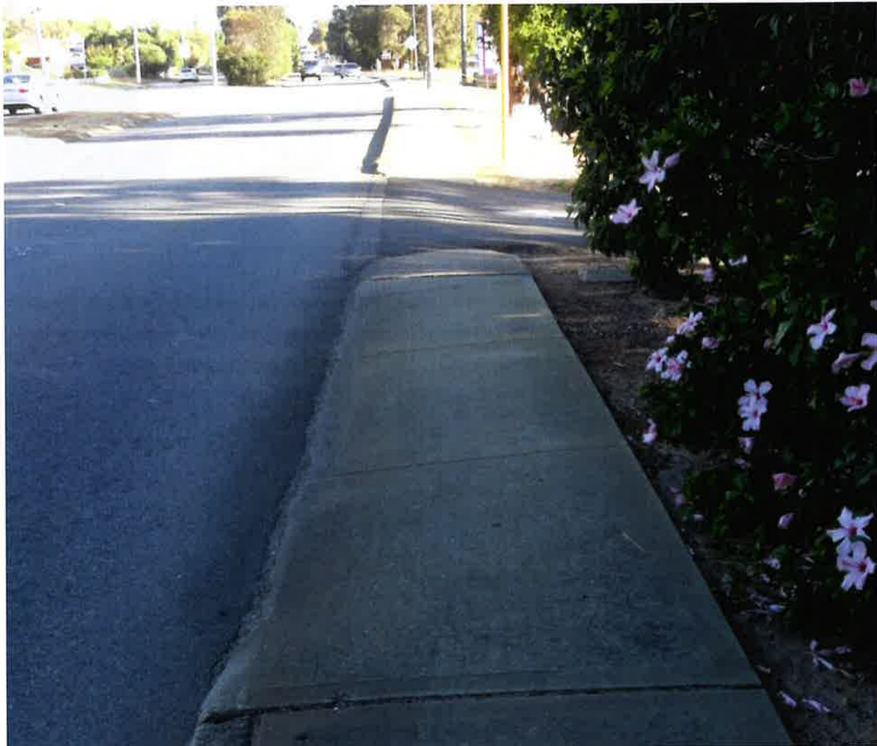
Photograph 15 – Example of South Western Hwy path on west side sloping towards traffic
