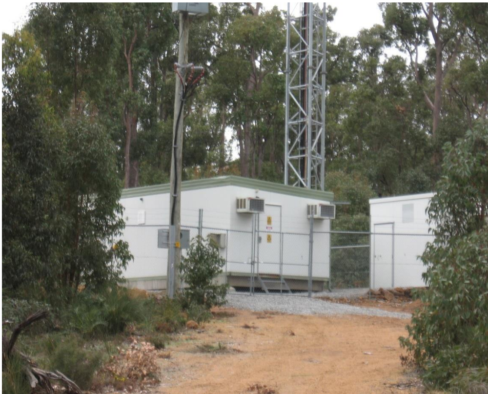
(Site Image: Tower & Infrastructure)
