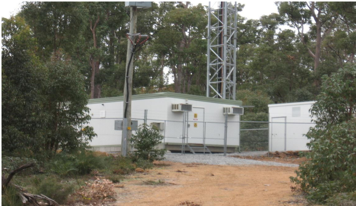
(Site Image: Tower & Infrastructure)
