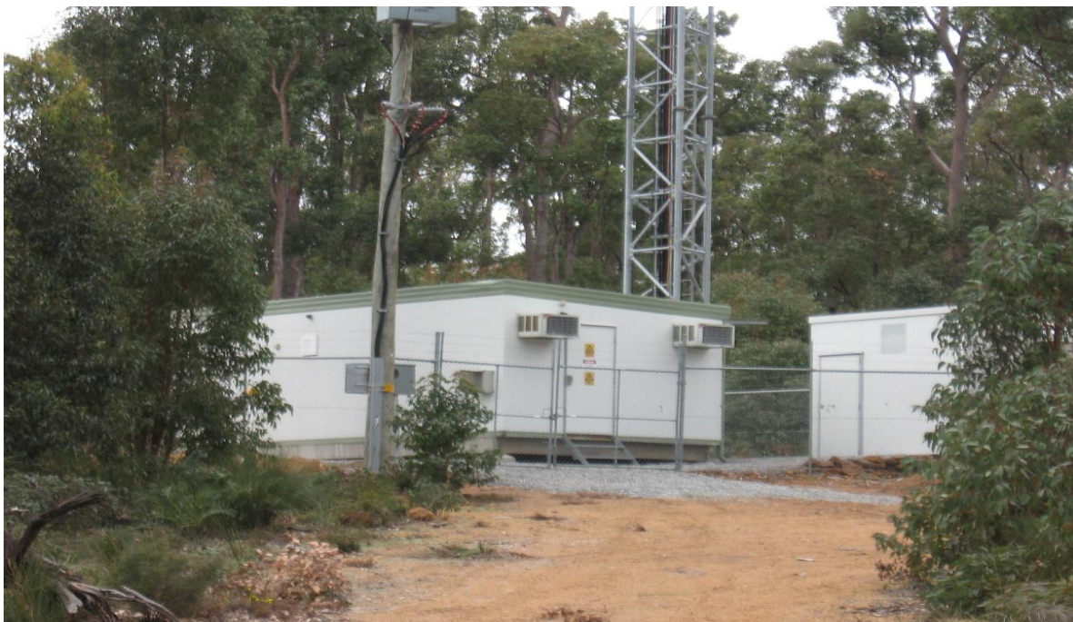
(Site Image: Tower & Infrastructure)
