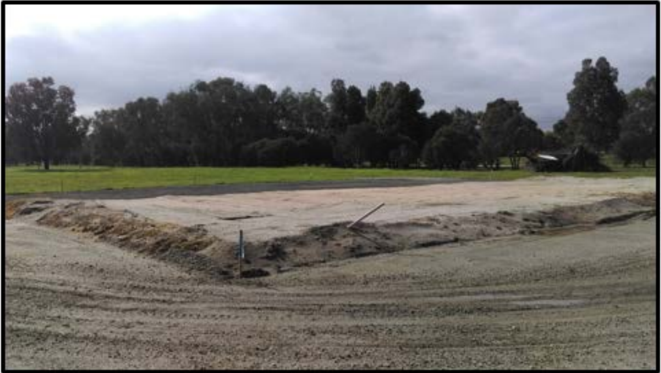
Figure 6: Viewing the extent of the fill from the south-western corner of the property.
