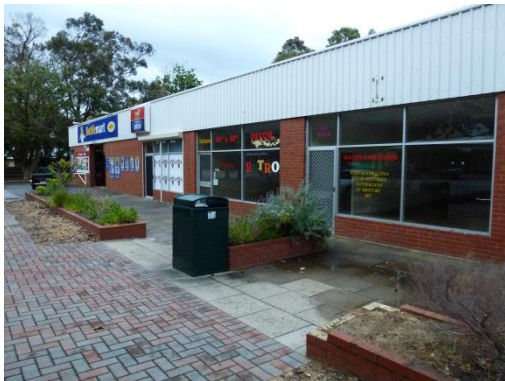
Figure 31: The brick wall surrounding the garden bed appears damaged and requires rectification
