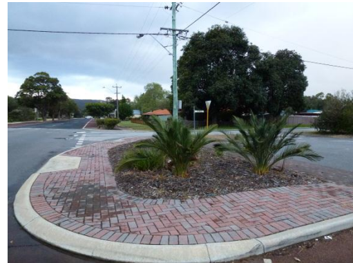
Figure 28: Brick paving appears dated and requires rectification to enhance a sense of ownership for the community
