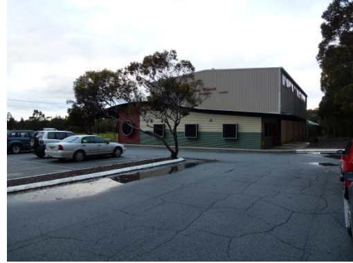
Figure 18: Car park appears dated and requires resurfacing
