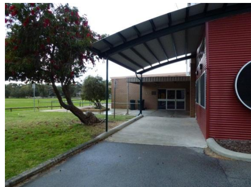
Figure 22: Entrance to Recreation Centre receives poor natural surveillance from car park and surrounding areas
