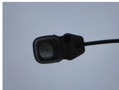
Figure 1: Sample street lighting used in Mundijong
